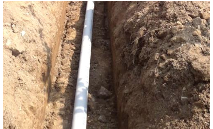
A New 2inch Water Connection line
